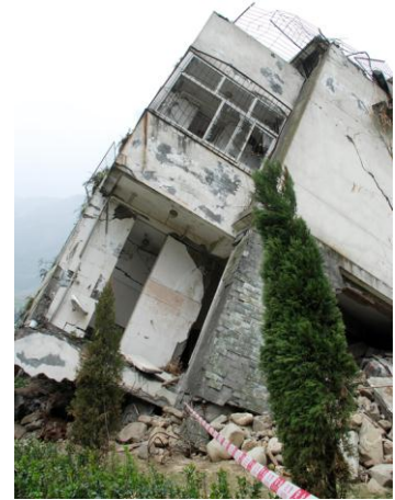
Magnitude 7.9 Earthquake Damage Sichuan, China 2008 © Hupengi | Dreamstime.com
